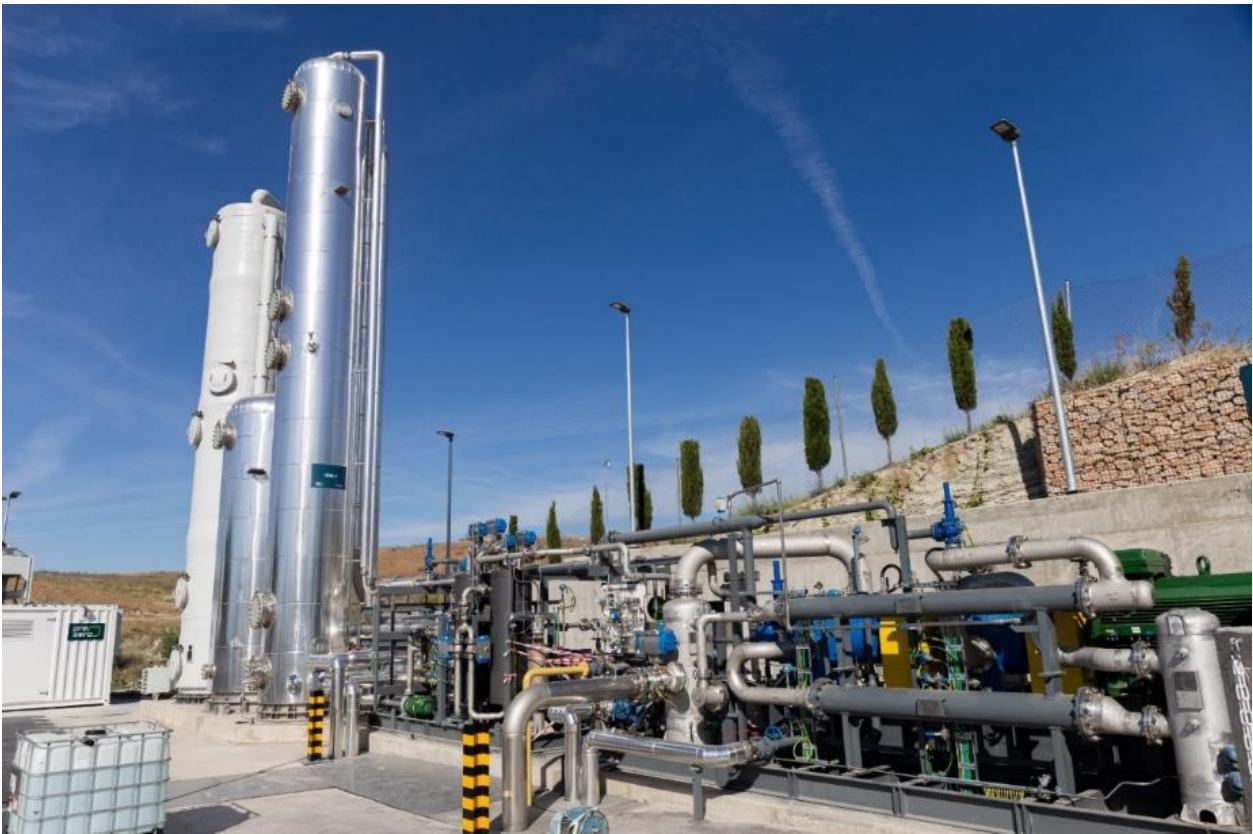
Biogas treatment plant extension
